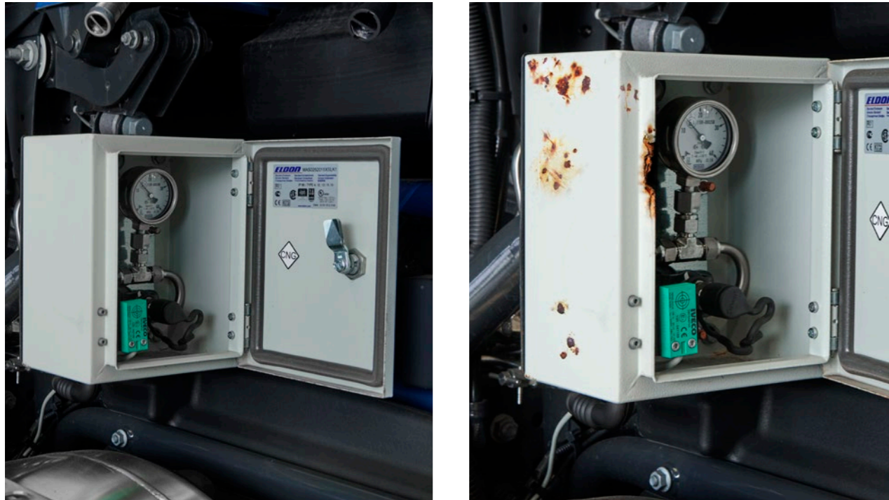
Rust on the fill receptacle protection box → note without charge for damage.
