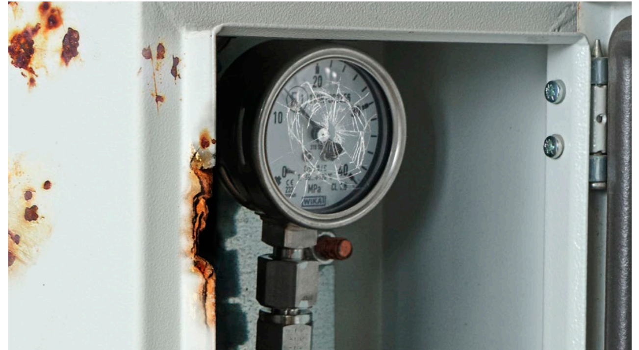
Missing protection box key, damaged CNG receptacle or pressure gauge → charge for replacement of the full box.
