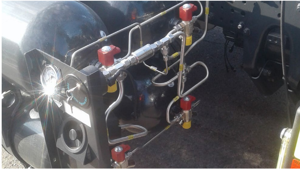
CNG cylinders must be returned in proper conditions as illustrated in picture.
