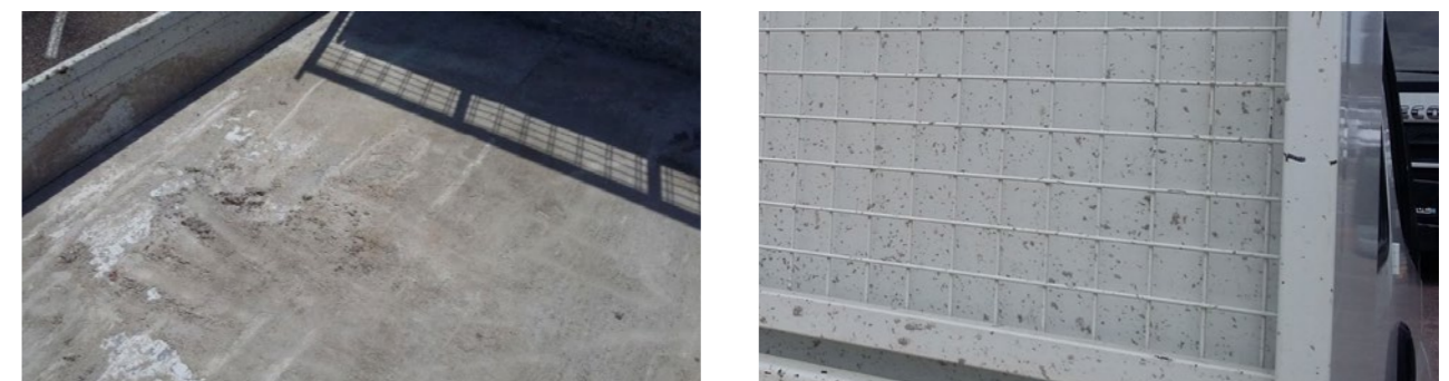
Trace of concrete or chemical product covering \geq 1/4 of the surface of the hopper
